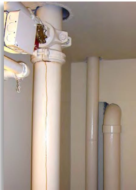
The walls of this fire-rated exit stair enclosure have been compromised by a plastic drain, waste, and vent pipe.
