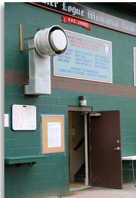
The distance between the exhaust point from this commercial cooking system and the operable door should be confirmed for compliance with national standards. Photo courtesy of Keith Heckler, Rockville Fire Department, Maryland.
