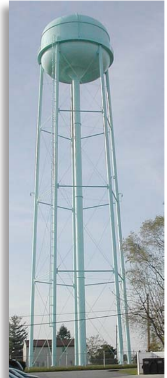
The water in this elevated supply tank is susceptible to freezing and should be provided with a heating source.
