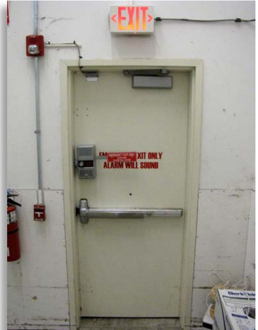
This exit door has too many hardware devices on it to comply with the model fire codes. Photo courtesy of Tim Mier, Cuyahoga Falls Fire Department, Ohio.
