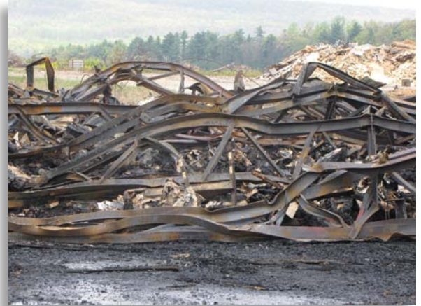
This pile of twisted steel is all that remains of a noncombustible building that was destroyed by a fire.
