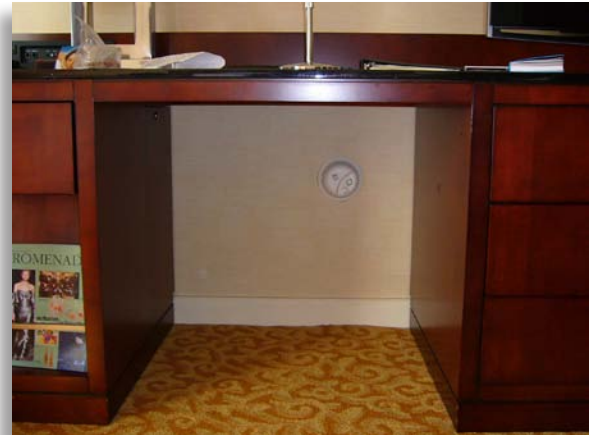
The location of this carbon monoxide detector acknowledges the specific gravity of the toxic gas.
