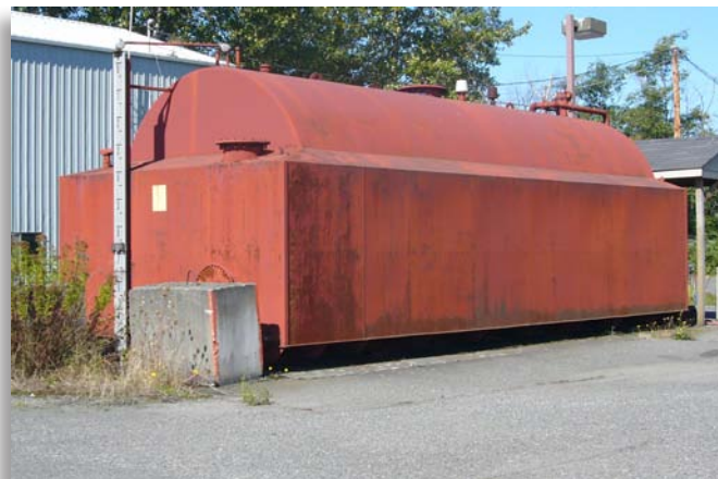
This horizontal tank is outfitted with a secondary containment enclosure for built-in spill capture.
