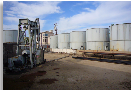
The storage tanks at this drilling site are uniform in size, so they will have the same wetted area and vent capacities.
