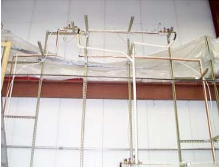
Figure 3. Partial piping system showing PEX and copper distribution systems, drains, and outlet measurement systems
