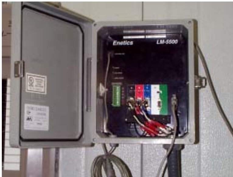
Figure 9. Power meter used to measure water heater energy use
