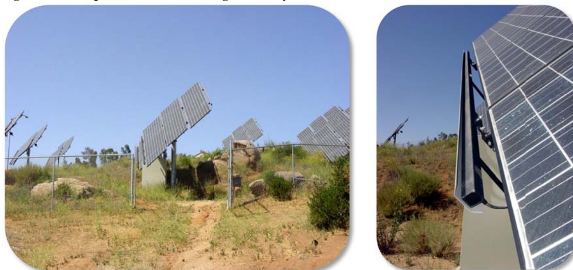
Figure 7. Example of Passive Tracking PV Array
