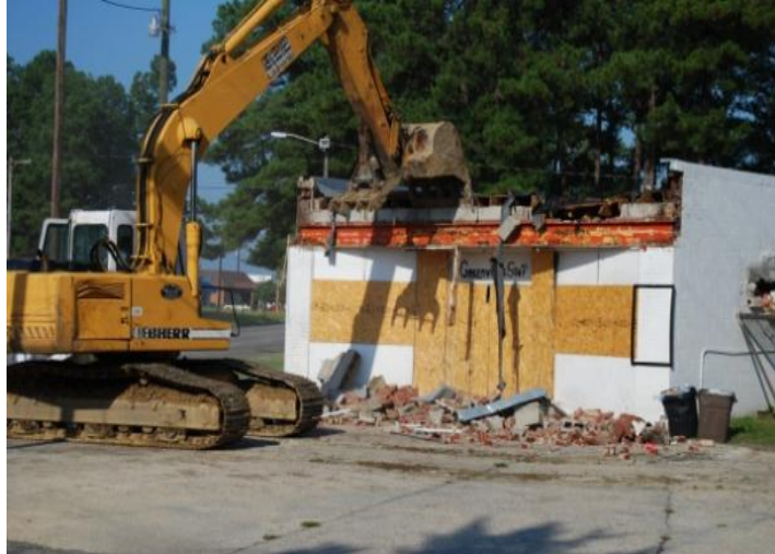
(1) Store in Greenville, NC being demolished to prevent the possibility of illegal activities resuming at the site. Greenville, NC Police Department Photo.
