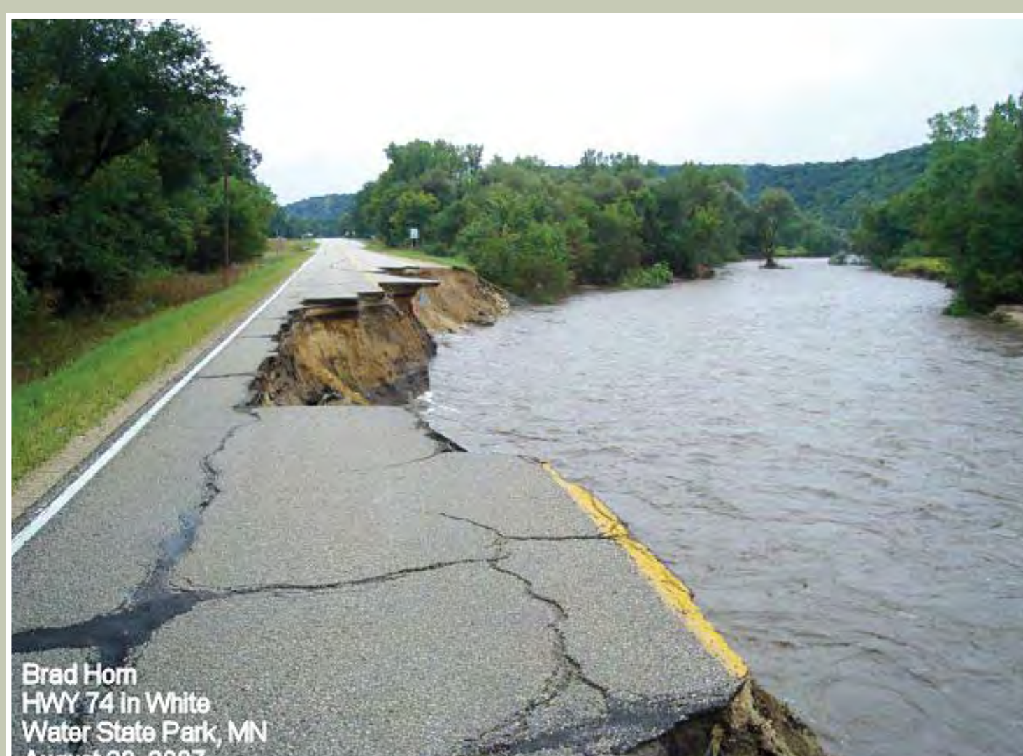
Highway erosion along Whitewater River, Minnesota (courtesy of National Weather Service)
