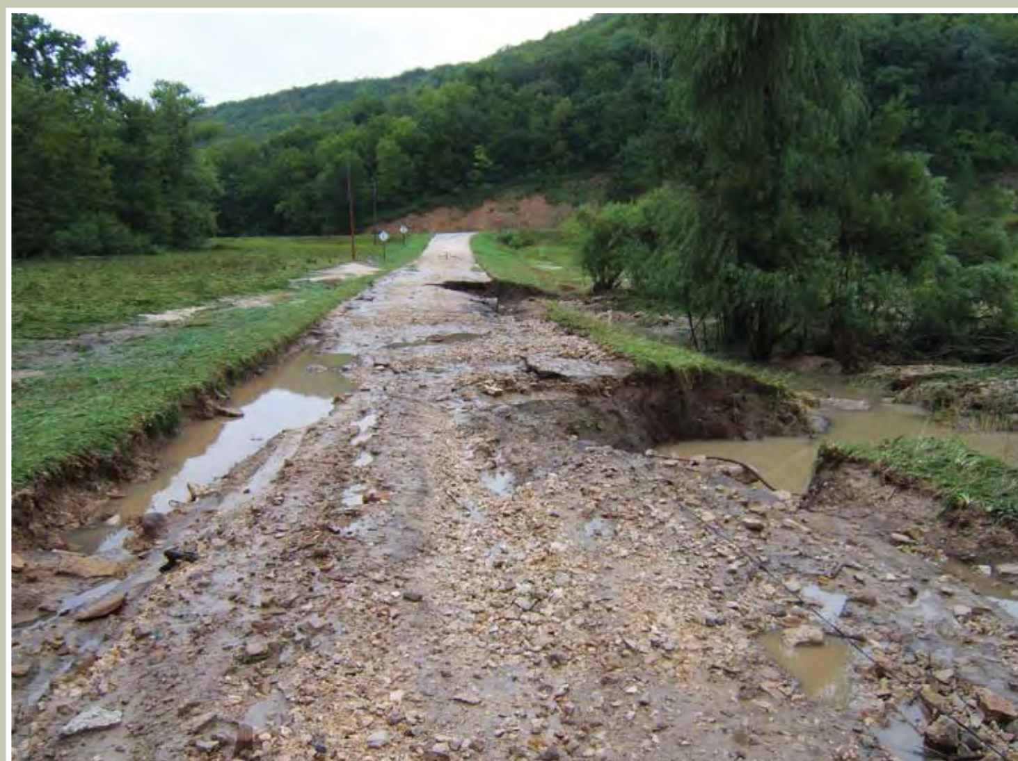
Washed out roads adjacent to Cedar Creek, Minnesota
