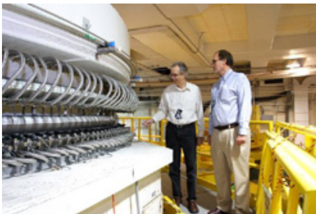
FIGURE 2: Tony Norbedo and Paul Brand inspecting headers of the thermal shield cooling system.
