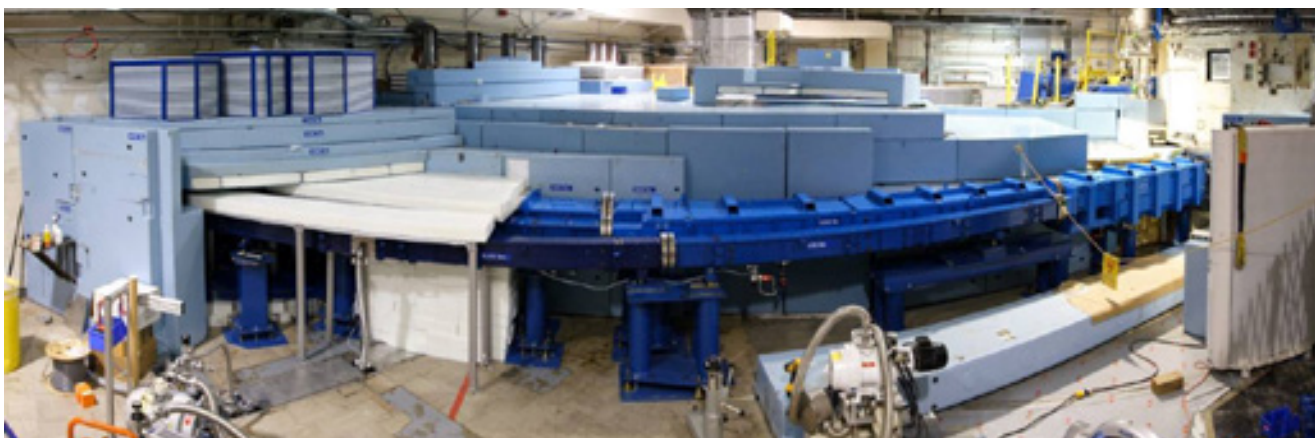
FIGURE 6: A view of the new guides and shields in the latter stages of installation in the confinement building, coming from the reactor on the right and entering D-wing on the left. (The apparent curvature is an artifact arising from the fisheye-lens camera.)
