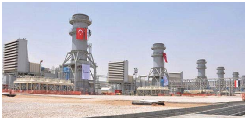
The 1,250 MW al-Qaryat power plant in Kerbala was completed in April 2013, marking the first completion of a plant built around turbines the GOI purchased in the GE “Mega Deal.” (Çalık Enerji photo)
