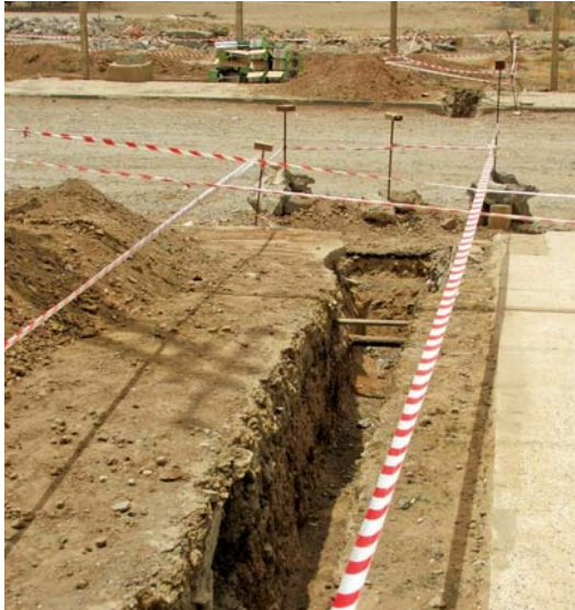
Pipework at the Hammam Al Alil Regional Training Center.
