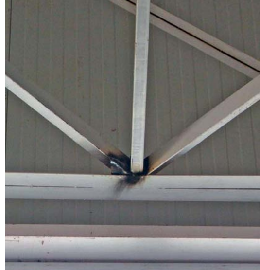
Inferior welds at the Abu Ghraib Dairy.
