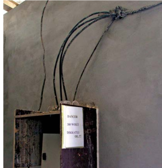
Faulty electrical wiring at the Rabeaa Point of Entry.
