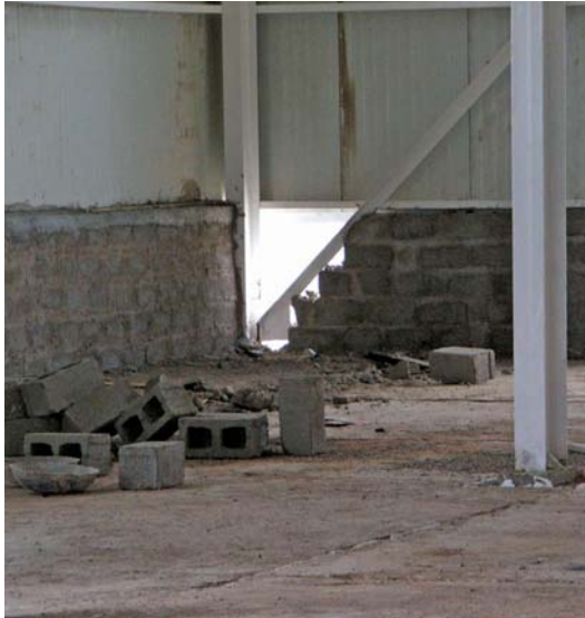
Improper masonry work at the Abu Ghraib Dairy.
