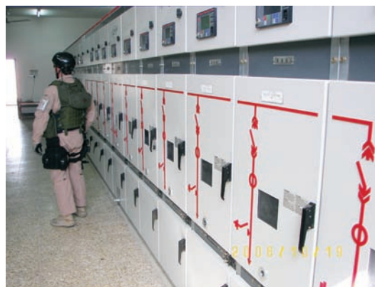
Site Photo 27. Al Hamdan substation distribution: 11 kV switchgear panels at the time of the second assessment.
