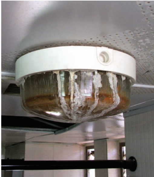
Site Photo 21. Urine-filled ceiling light.
