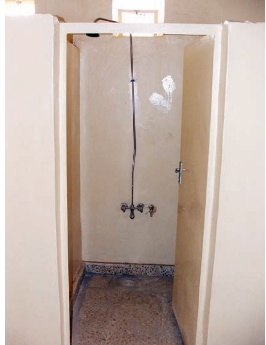
Site Photo 14. Shower facilities at the 2nd Brigade garrison showing a thin wall metal tubing shower fixture connected to the wall with a single screw clamp.
