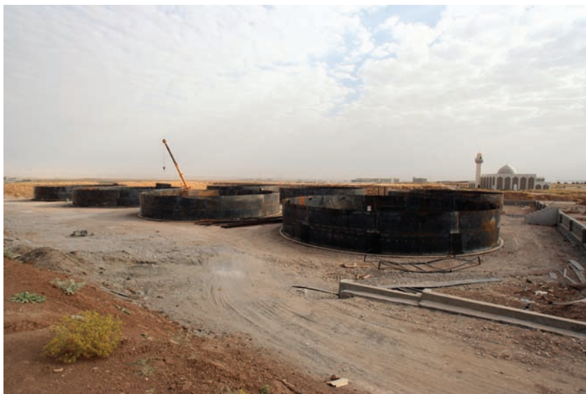
Site Photo 10. Overall progress of water storage tank construction, as of August 1, 2006.
