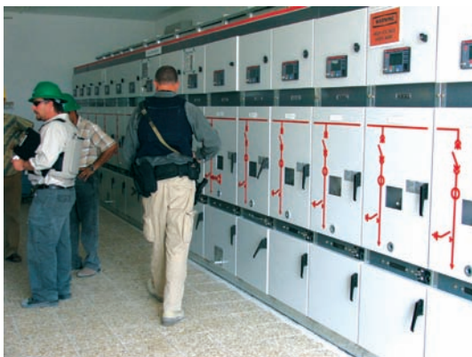
Site Photo 26. Al Hamdan substation distribution: 11 kV switchgear panels at the time of the initial assessment.
