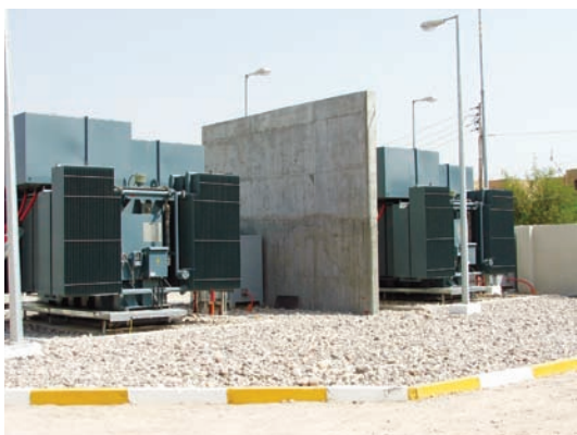
Site Photo 28. Al Serajii 33/11 kV transformer, first assessment.
