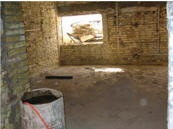
Site Photo 3. Patient ward in Building B9 after demolition of wall plaster and flooring.
