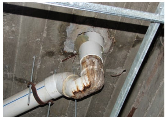
Site Photo 20. Effects of wastewater leaking on plumbing pipes.
