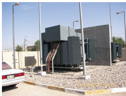
Site Photo 29. Al Serajii 33/11 kV transformer, second assessment.
