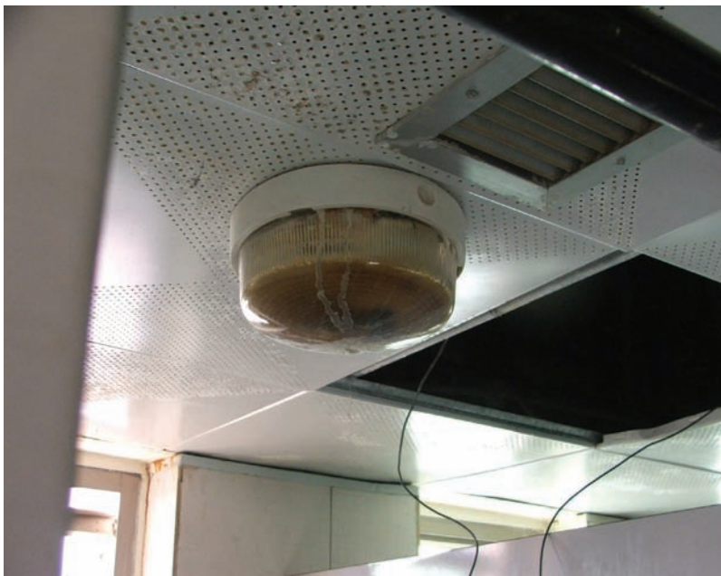
Site Photo 22. Urine-filled ceiling light and hanging wires.
