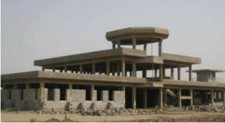
Khan Bani Sa'ad Correctional Facility abandoned after approximately $40 million had been spent. (GRD photo)
