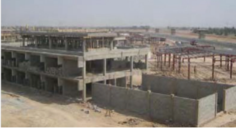
Incomplete building at Khan Bani Sa'ad Correctional Facility, 2006.
