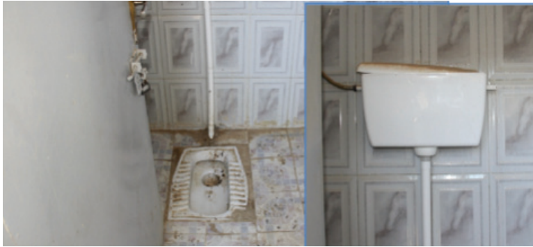
Bathroom with no running water in a school built in Anbar province with CAP funds, February 2011.
