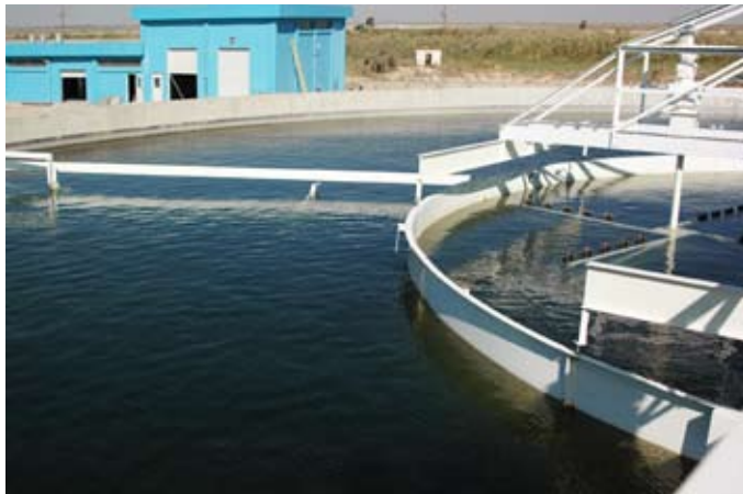
Refurbished water treatment plant.
