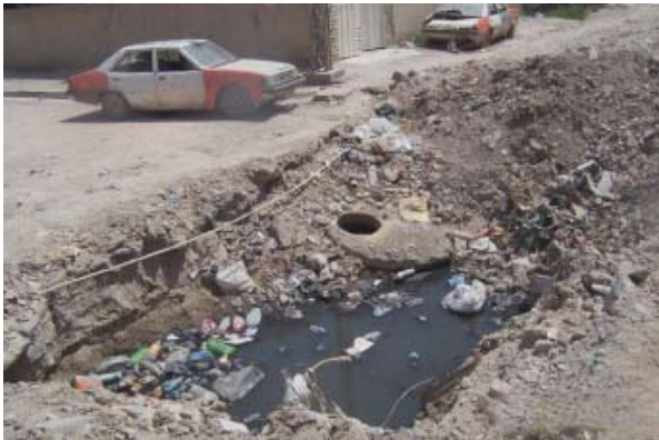
Collapsed existing manhole before construction completed by the contractor. (Photo courtesy of USACE)
