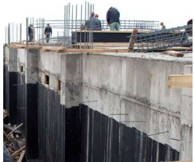
Throughout the facility, exposed concrete finish was smooth, with no sign of excessive material separation during casting. Also, per the Scope of Work, below-grade concrete was waterproofed.
