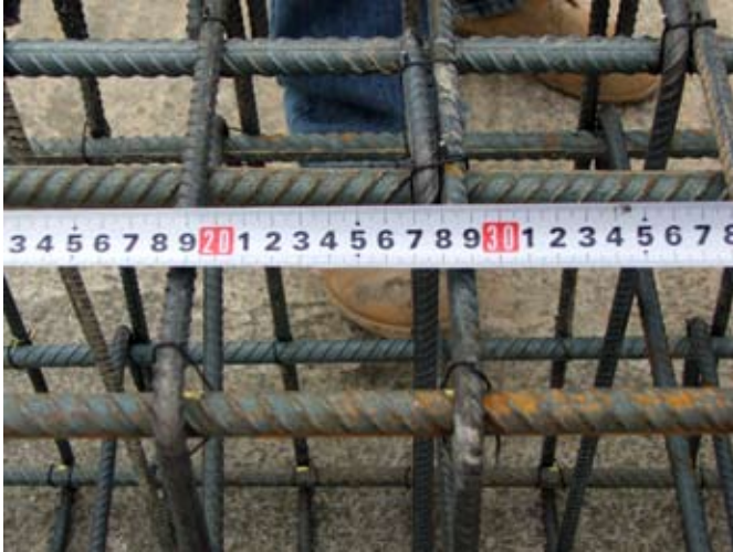
Rebar was pre-measured and marked to facilitate correct placement of rebar assembly components.
