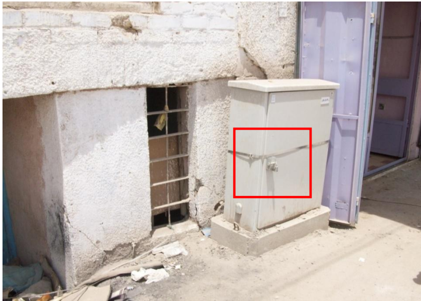
Figure 3—Banded and Locked Pillar
