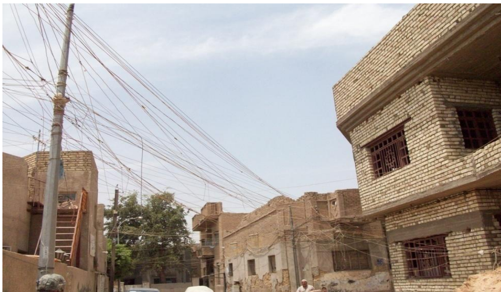
Figure 4—Resident-Installed Electrical Lines in Muhalla 312
